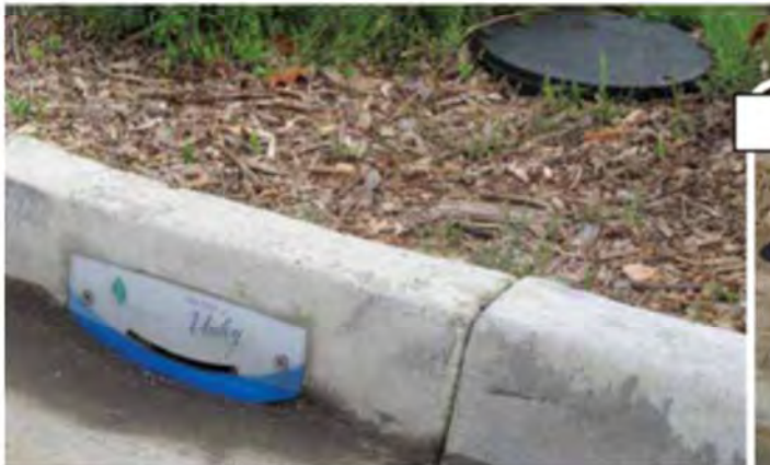
TreeNet inlets capture stormwater from water runoff and utilise the water to support tree growth.
